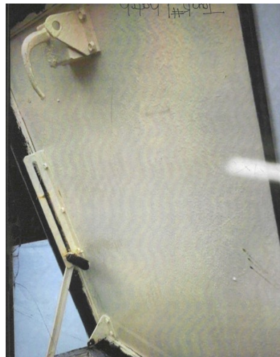
Reservoir #1 hatch seal
