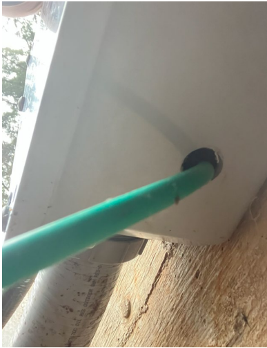
Well #2's junction box not sealed at the conduit connection
