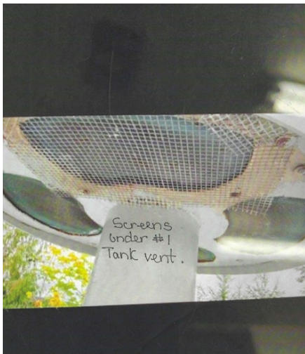
Reservoir #1 vent screens
