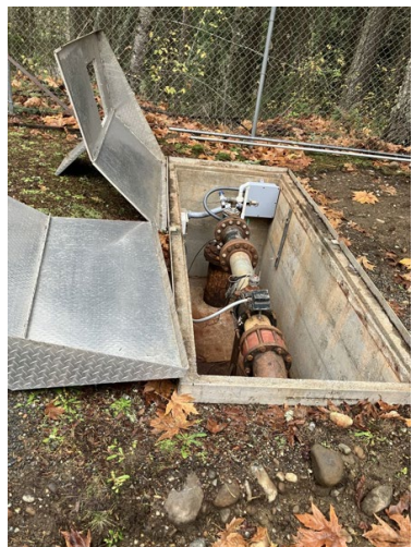
Well #2's vault
