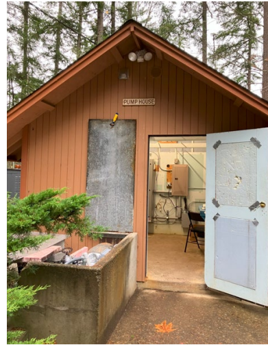
Well #1 Pump House, disconnected
