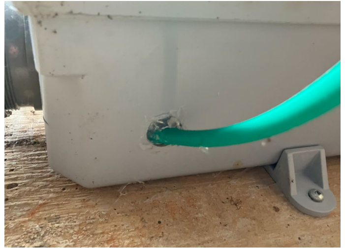
This was sealed with silicon at the survey
