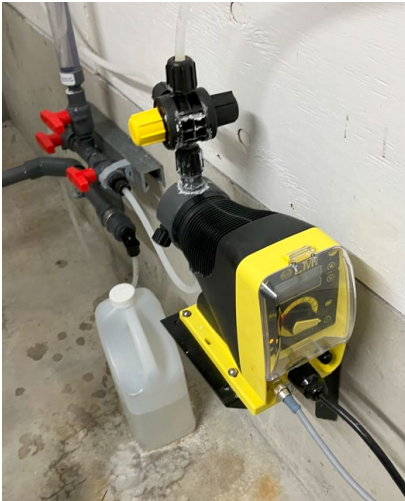
Caustic soda injection pump
