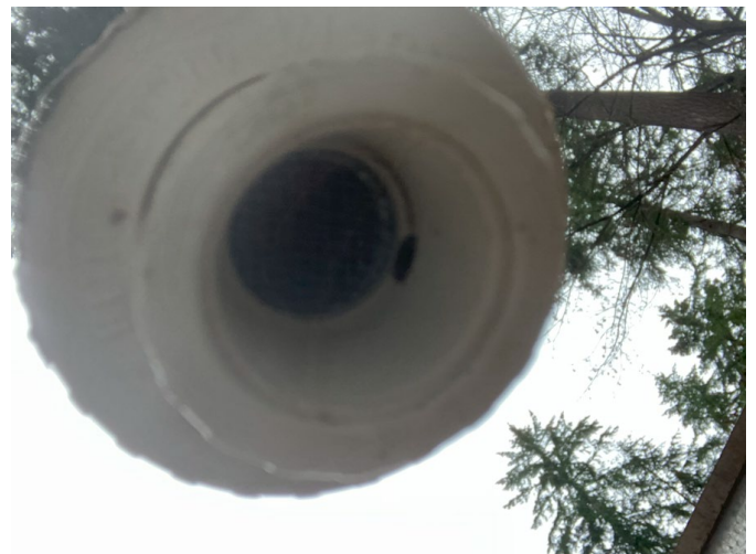
Well #2's vent screened
