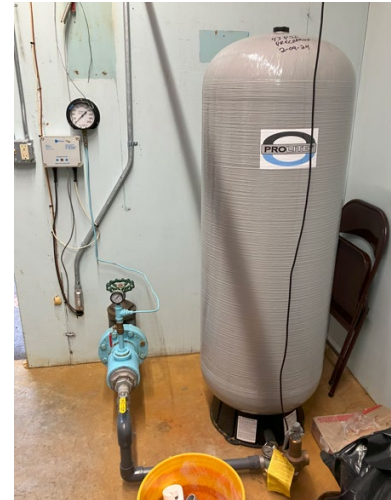
Well #1 Pump House's new bladder tank, disconnected
