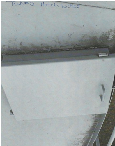
Reservoir #2 hatch locked
