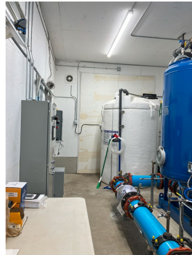
Caustic soda tank
